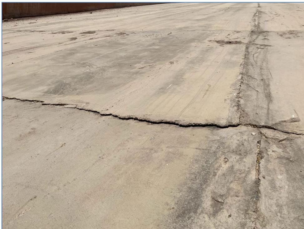
Figure 3:Bad Joint Arrangement Just After Construction.
