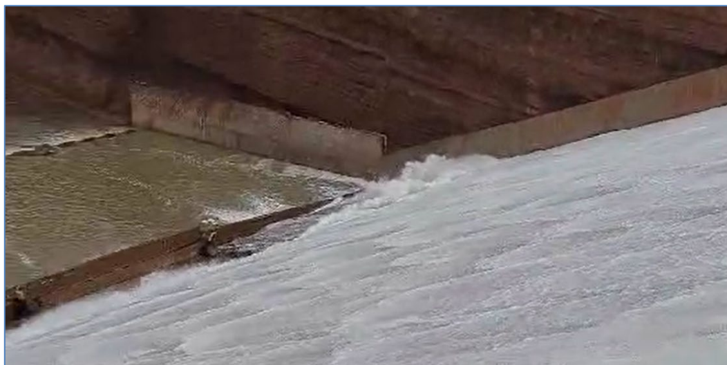
Figure 4:Photo Showing Some Displaced Panels.
