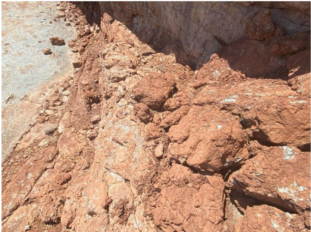
Figure 10: Weathered rock beneath the chute slab of the Dewan Dam spillway.
