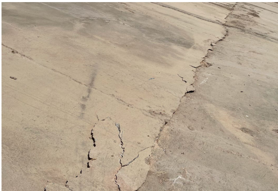
Figure 7: Cracks and bad joint finishing
