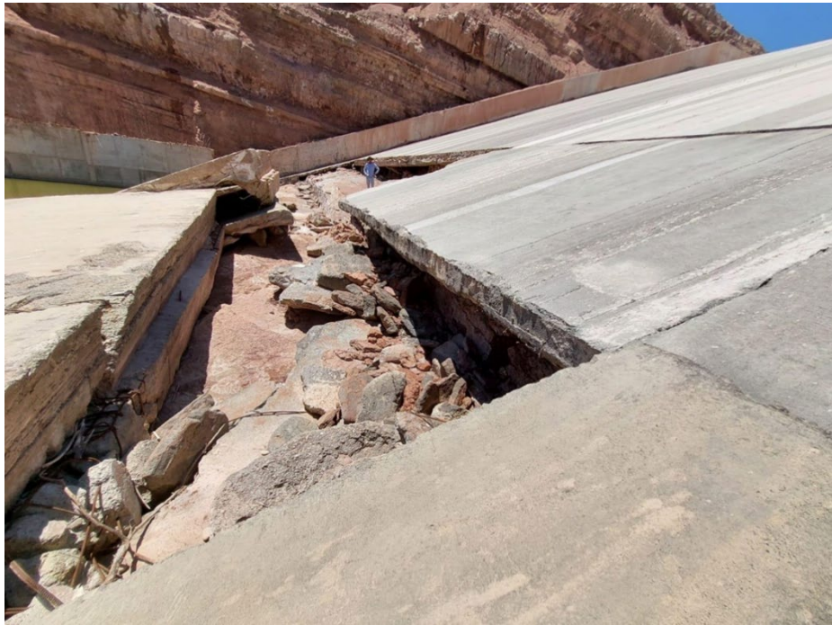
Figure 11: Poor quality rock beneath the chute slab of the Dewan Dam spillway.
