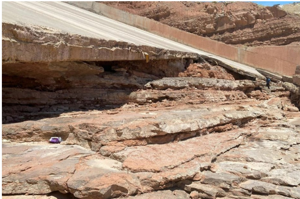
Figure 5: Exposed foundation showing thin jointed beddings downstream.
