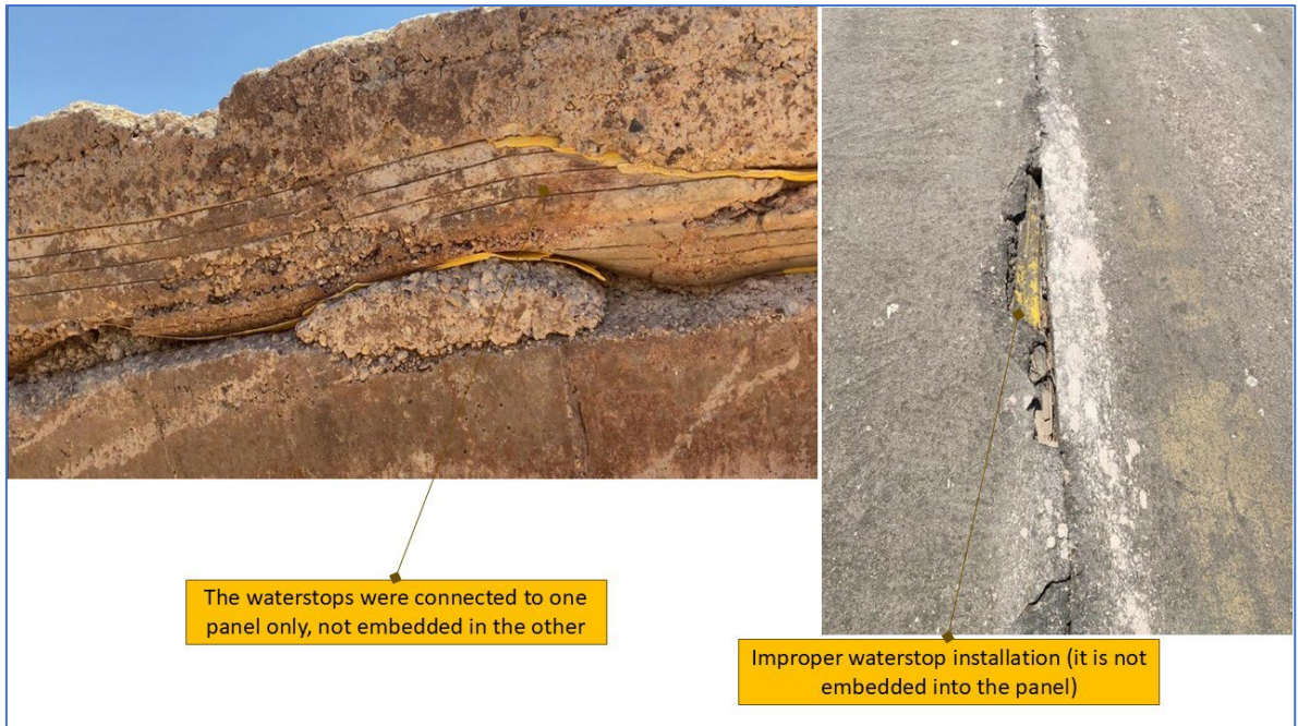
Figure 9: Improper waterstops installation.
